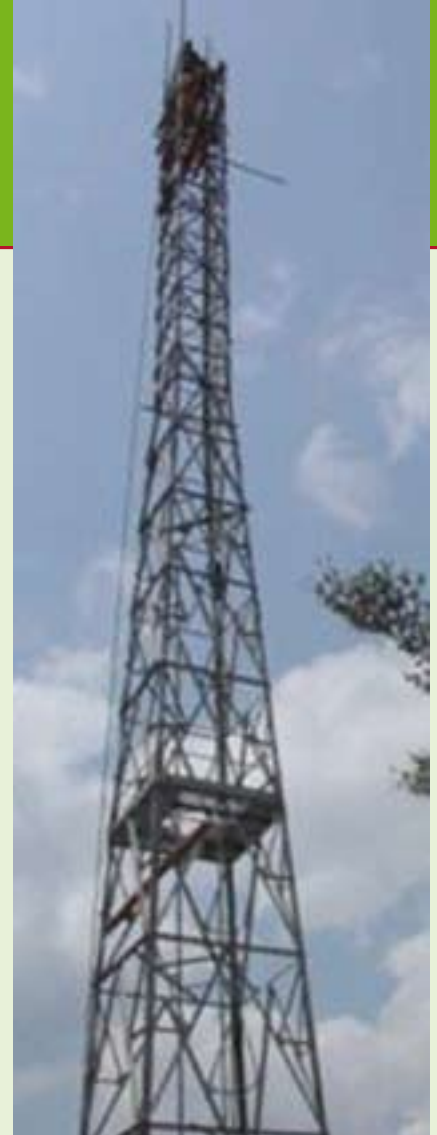
30-Meter-Antenne des Senders Maendeleo
