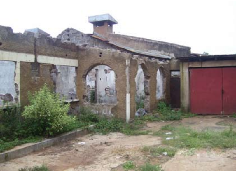
The remains of a vandalized house after the post election violence
