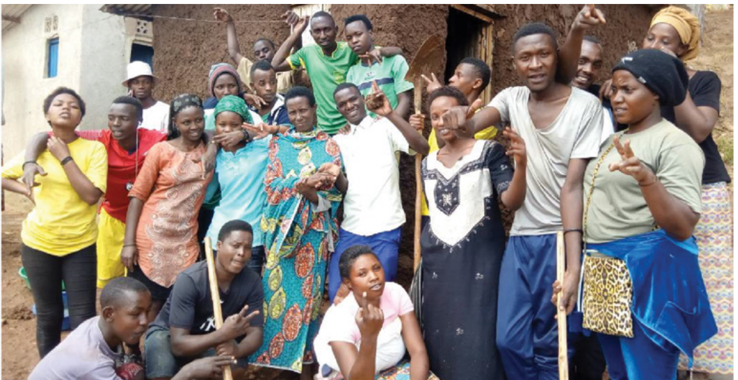
Pic: Youth from Mugombwa refugee camp and host community after rehabilitating a house for a community member
