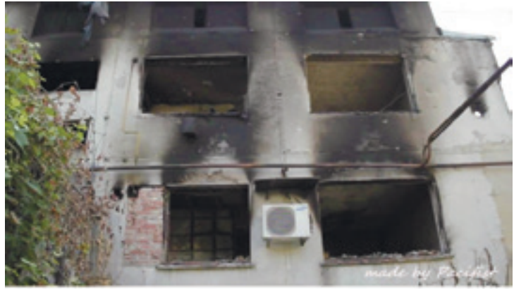
Destroyed house in Maryinka (Donetsk Oblast), 2015. Photo credit: local resident L., who wished to remain anonymous
