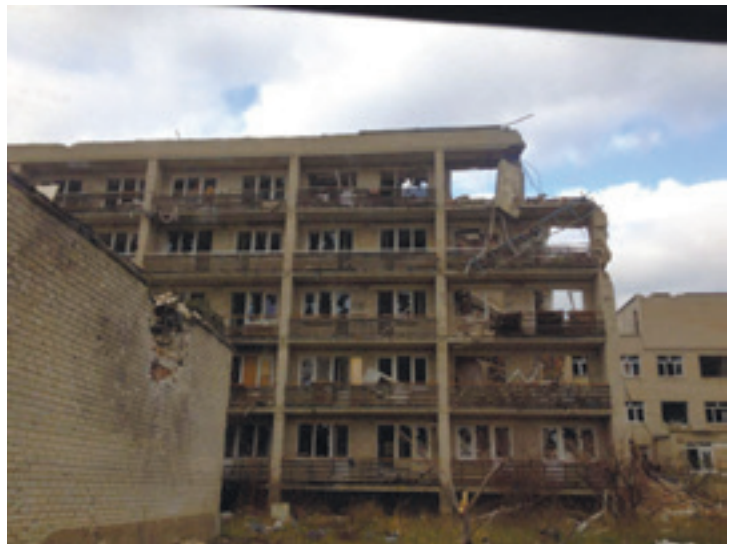
Damaged school dormitory in Maryinka (Donetsk Oblast), 2016. Photo credit: Denys Kazanskiy 24
