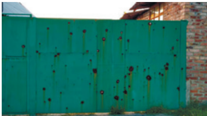
Fig 4. Private home gate damaged by shrapnel, 91 Shevchenka Street, Bakhmut, 18 September 2017, photo credit: M. Bilyakova.
