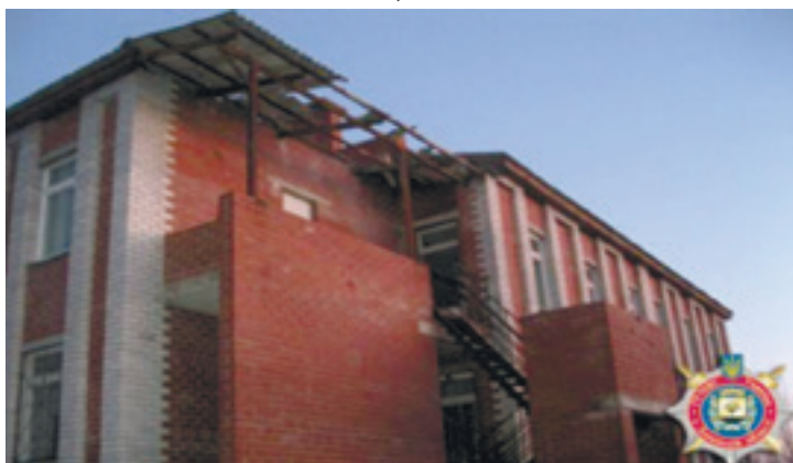
Fig. 1. The damage to "Lelechenka" kindergarten building, 22, First Zahorodnya Street, Bakhmut, 13 February 2015, photo credit: MIA in Donetsk Oblast 2
