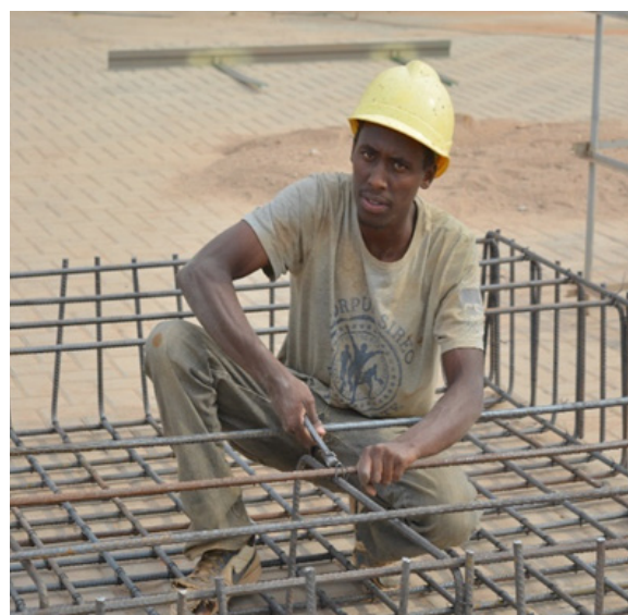
GASHEJA NSENGIYUMVA is now skilled in bending steel bars; here he was at a petrol station under construction at Gishushu in Kigali (Photo, Kigeme Iwacu)
